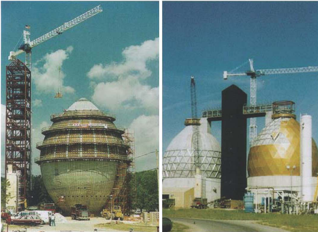
Baltimore, Maryland, USA. Two egg-shaped digesters 11,350 m 3 each.
